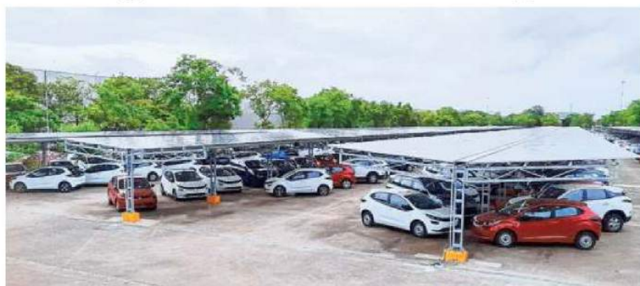
The 6.2 MWp solar carport will generate 86.4 lakh kWh of electricity per year and is estimated to reduce 7,000 tonnes of carbon emissions annually and 1.6 lakh tonnes over its lifecycle
